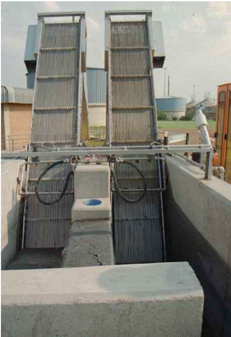
Figure A-8 - Sludge fine screens before the digesters
