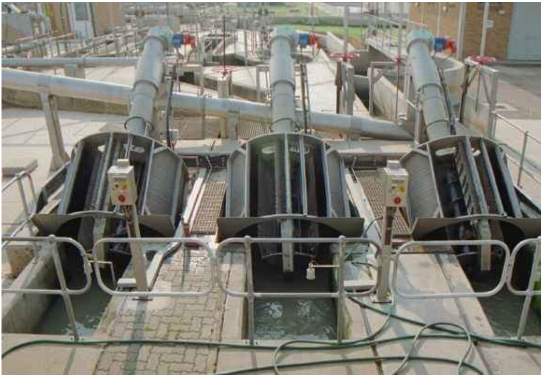
Figure A-5 - Rotating Disc Screens for the removal of coarse material from the flow stream
