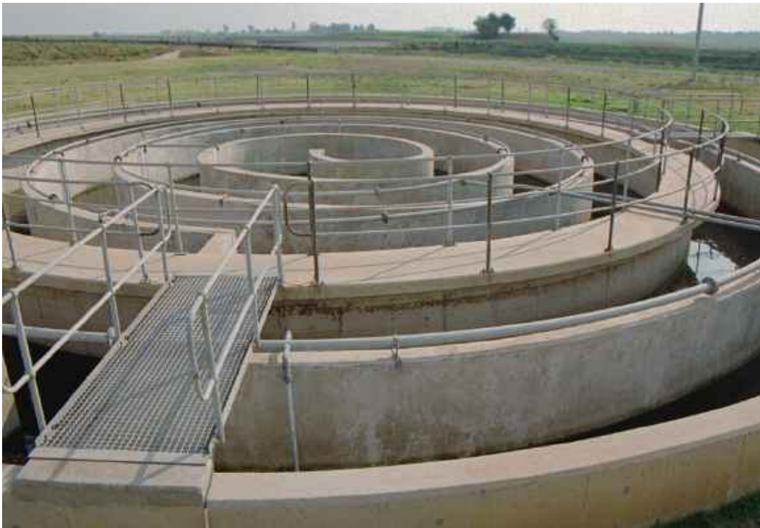
Figure A-7 - Chlorine Contact Chamber, which is used for disinfection purposes to destroy pathogenic bacteria
