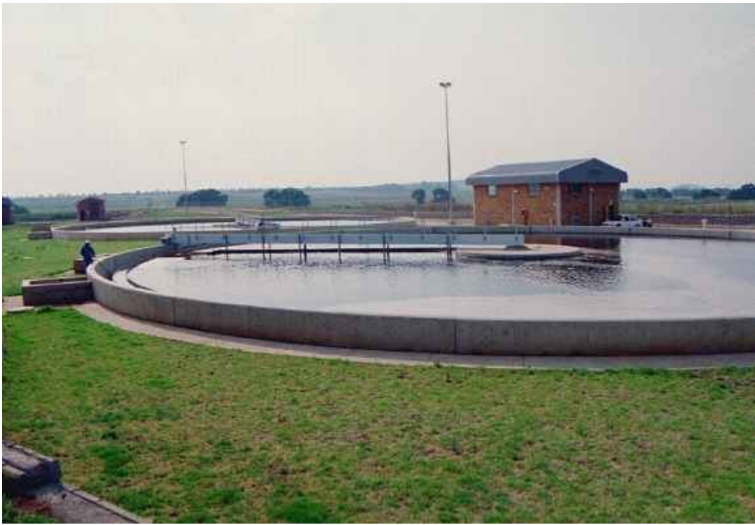
Figure A-7 - Secondary Settling Tank from another view
