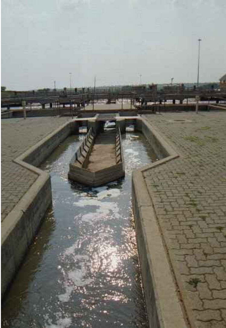
Figure A-3 - Settled sewage to the Bioreactor
