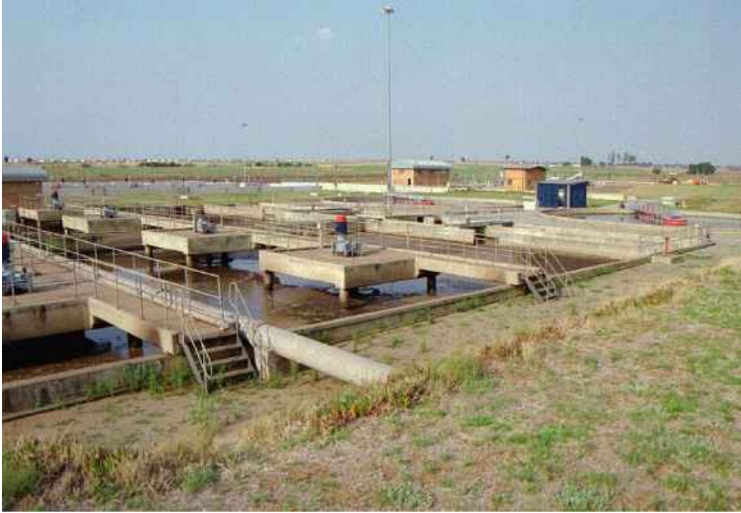
Figure A-4 - The main purpose of the bioreactor is to remove nutrients (nitrate, nitrite, phosphate, ammonia) from wastewater
