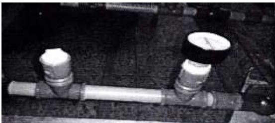
Fig. 3: Fixed pressure gauge
